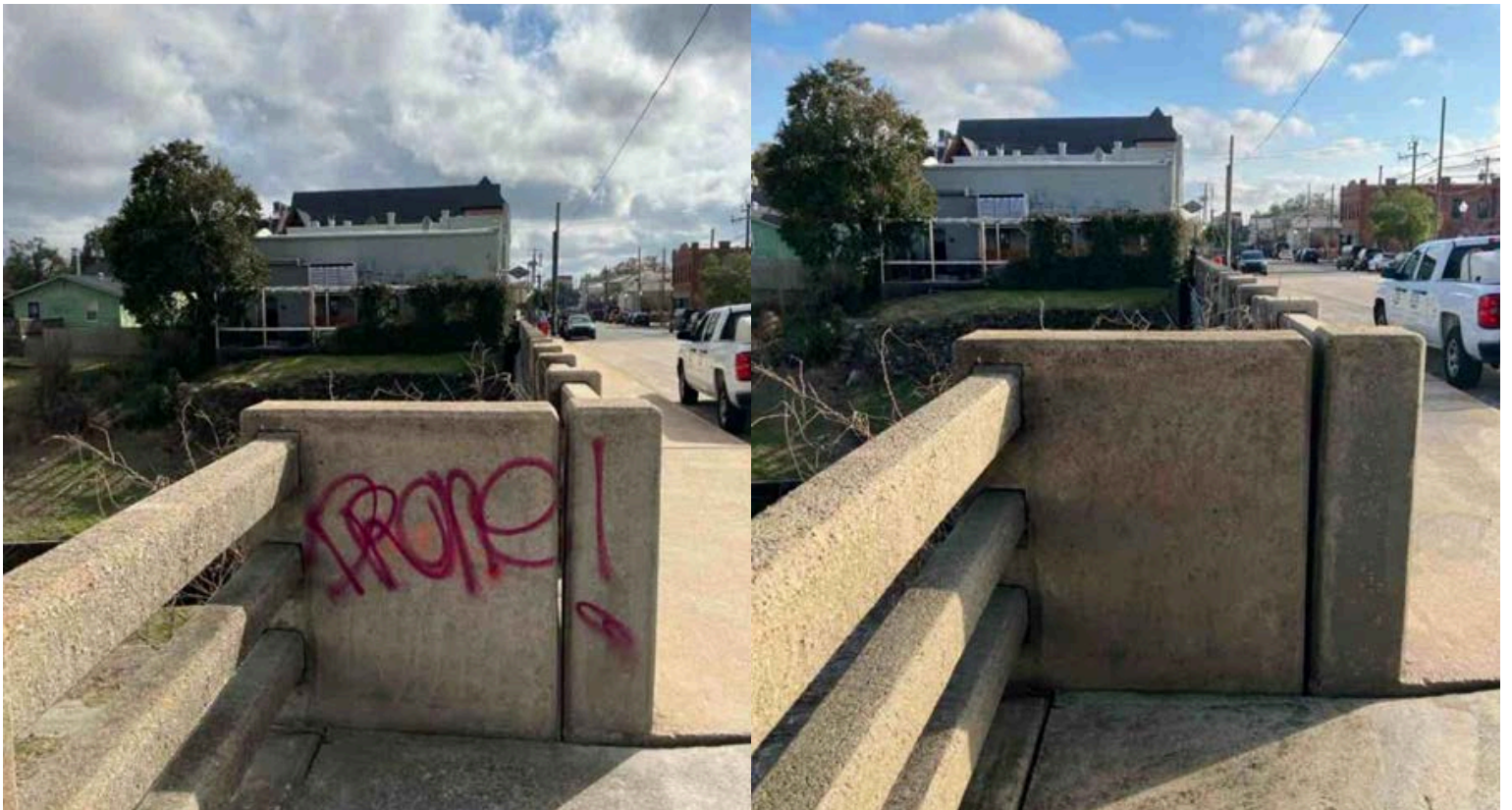
GRAFITTI REMOVAL – NORTH 4TH STREET
