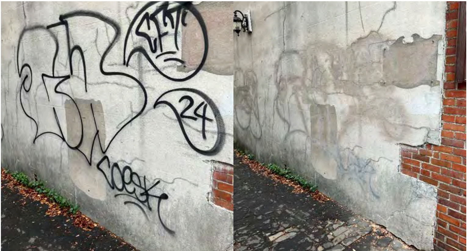
GRAFITTI REMOVAL – WILKINSON ALLEY
