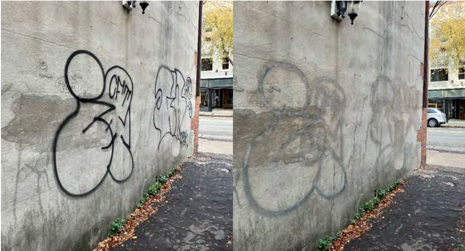
GRAFFITI REMOVAL – WILKINSON ALLEY
